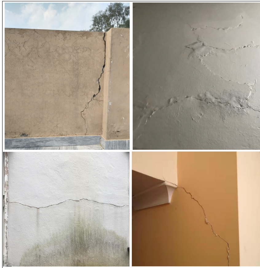
Figure 16. Building cracks due to ground subsidence in various places in Lahore City.
