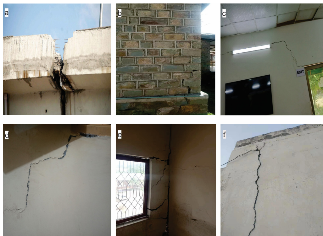
Figure 17. Cracks in the walls of different buildings within the research area. (a) Cracks in the pillars of metro track at Committee Chowk, (b–f) Cracks in walls of local houses in Raja Bazar, Waris Khan, Rehmanabad, and Sadiqabad areas.
